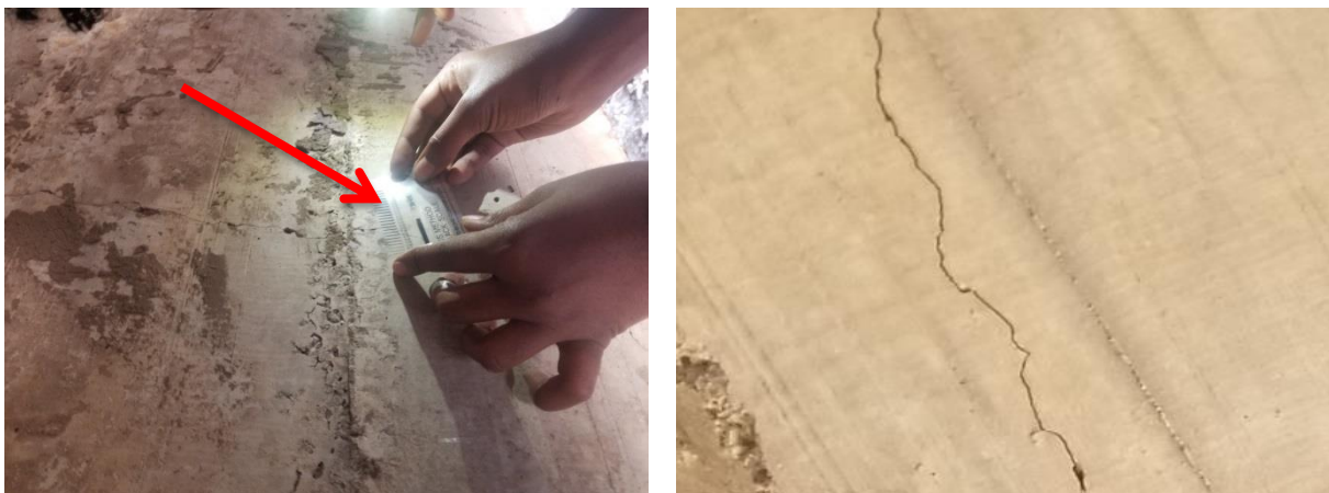
Figure 3. 4: Measuring the size of crack openings with crack scale
