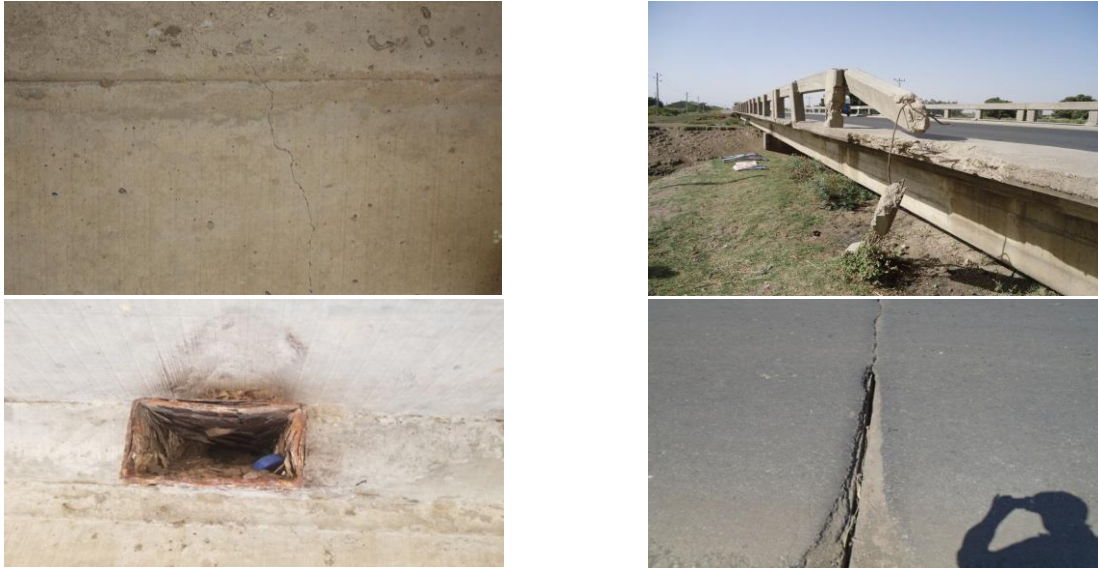
Figure 3. 5: Damage and Distresses on bridge super-structure.
