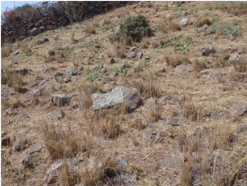
Plate 4.4 Highly fractured and disintegrated rock mass on right abutment
