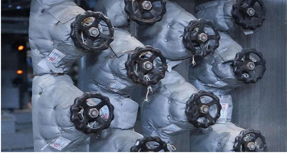
Figure 4-4 Insulation Jackets for flanges and valves
