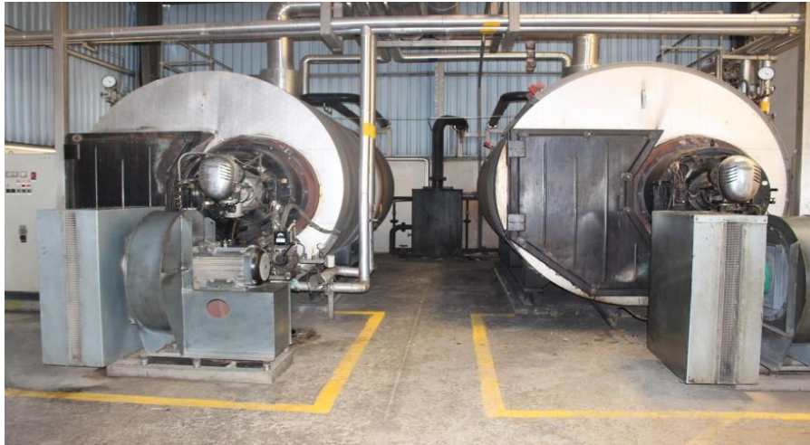
Figure 3.4 Fuel fired boilers of the factory
