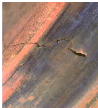
Figure 2.3: Fatigue crack on the Tread propagated from thermal crack
