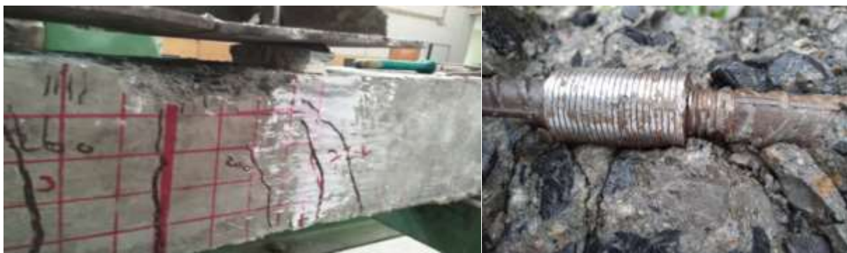
Figure 4-4: Mode of Failure for CIB-1
