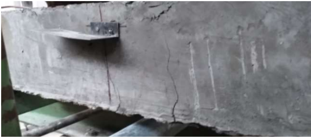
(C) Crack behavior of CIB-2
