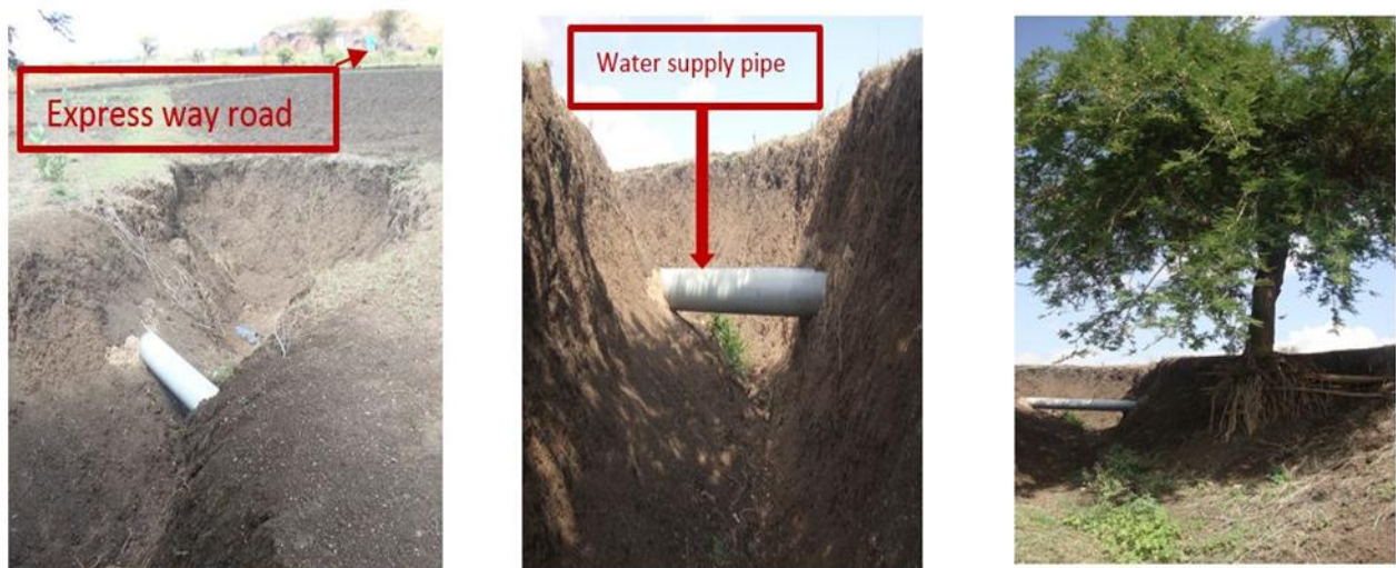
Figure 1. Flood is exposing water supply pipes & uprooting Acacia trees
