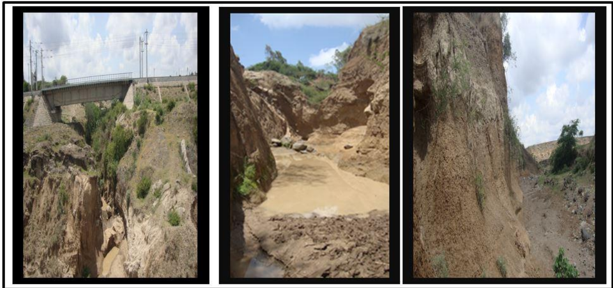
Figure 15. Pictures of Soil erosion around Moshe area
