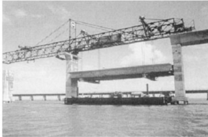
Figure 2.18: Lifting completed span of the Seven Mile Bridge, Florida, Using an overhead truss.
