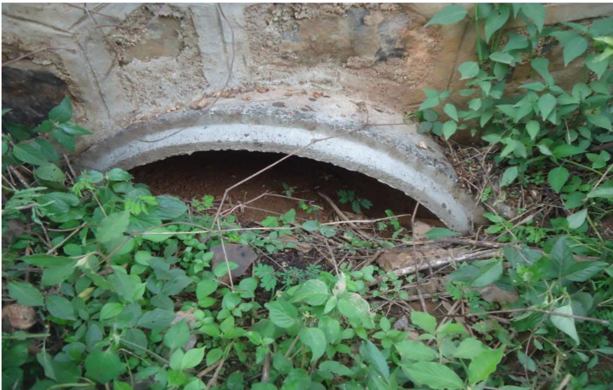
Figure 4.10 photo of Culvert taken from site Provision for adequate drainage is of paramount importance in road design and cannot be overemphasized. The presence of excess water or moisture within the roadway will adversely affect the engineering properties of the materials with which it was constructed. Cut or fill failures,
