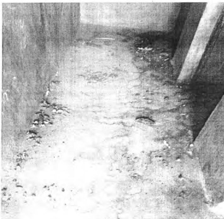
Figure 6: Dirty and smelly latrine with faeces on its floor in the Selamber school
