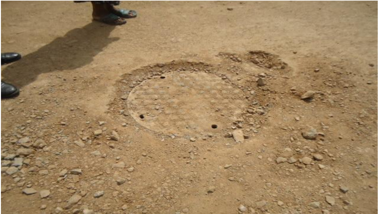
Figure 4.3 A sewer manhole around Berhanna Selam press (Photo taken on June, 2011)
