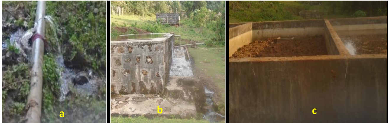
Figure 4-1: Picture showing water losses in conveyance and treatment units
