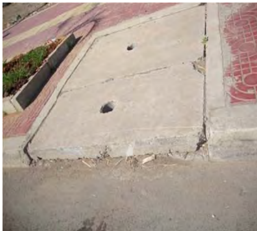
Fig 3.5 a) Inlet blocked by silt and garbage
