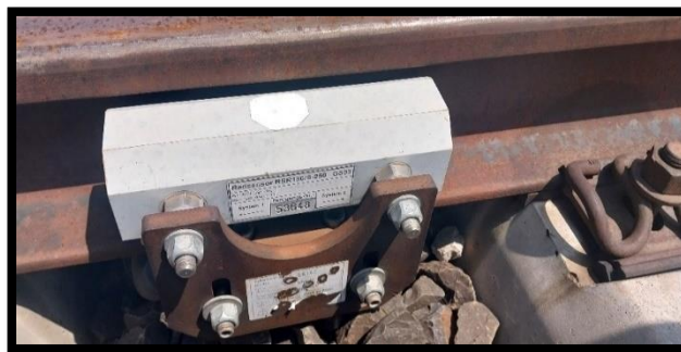
Figure 4.17: Axle counter placed on the railway track
