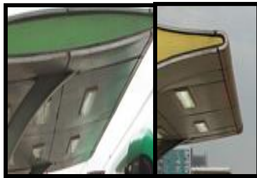
Figure 4.15: Station lights at the AALRT passenger platform
