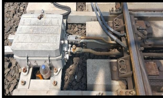
Figure 4.16: Point machine at Kality depot AALRT
