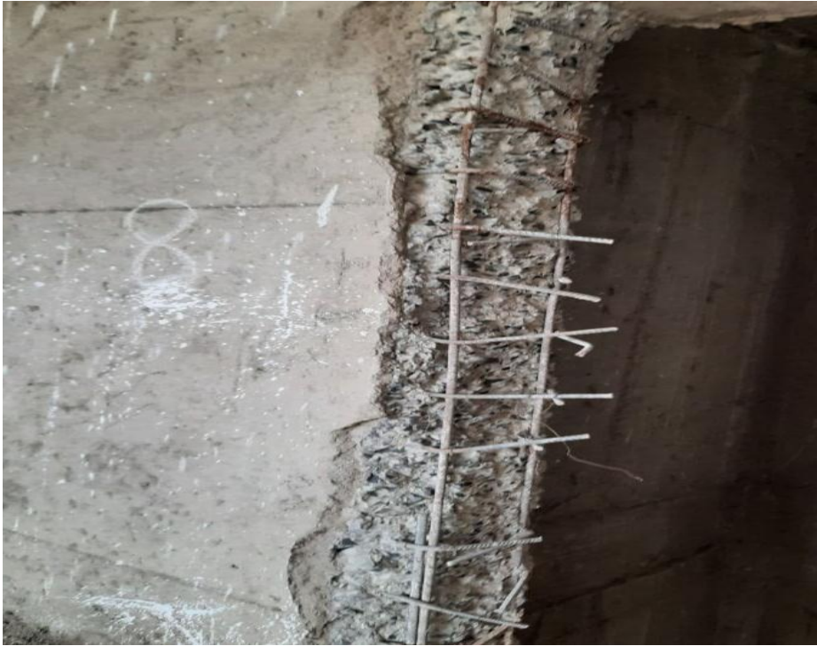
b) Defects on the lift shaft at bole bulbula project site
