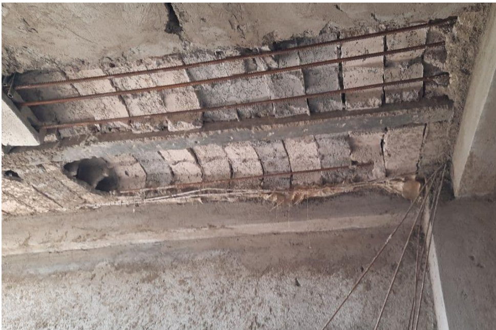
Figure 4.14 Rework due to poor quality of HCB at bole hayat project site
