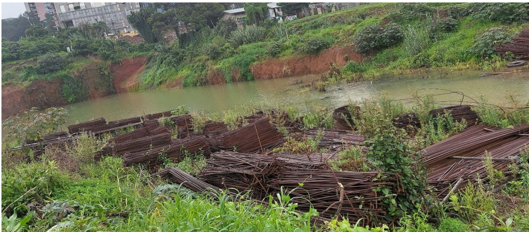
(a) Poor material storage system in leghar site
