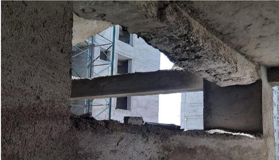
a) Defects on beams at bole beshale project site
