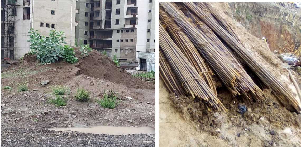
a) Sand stored in harsh weather in bole hayat site b) rebar stored in harsh weather in leghar
