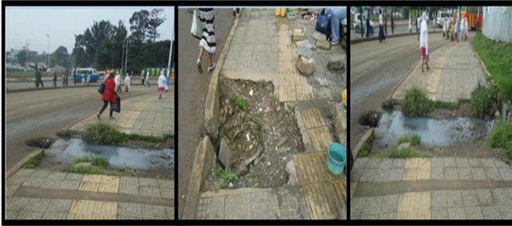
Figure 4-3: Cracked and unsafe pavement
