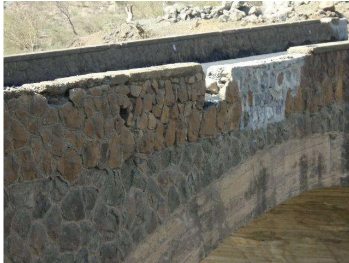
Figure 3-4 Damage by vehicle Collision on Parapet walls
