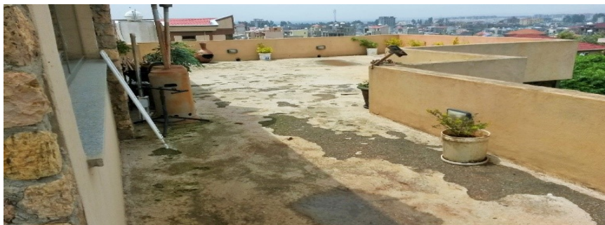
Figure 43 Unused vacant rooftop space on the same building, which can be used for further green roof expansion. Image source: site visit
