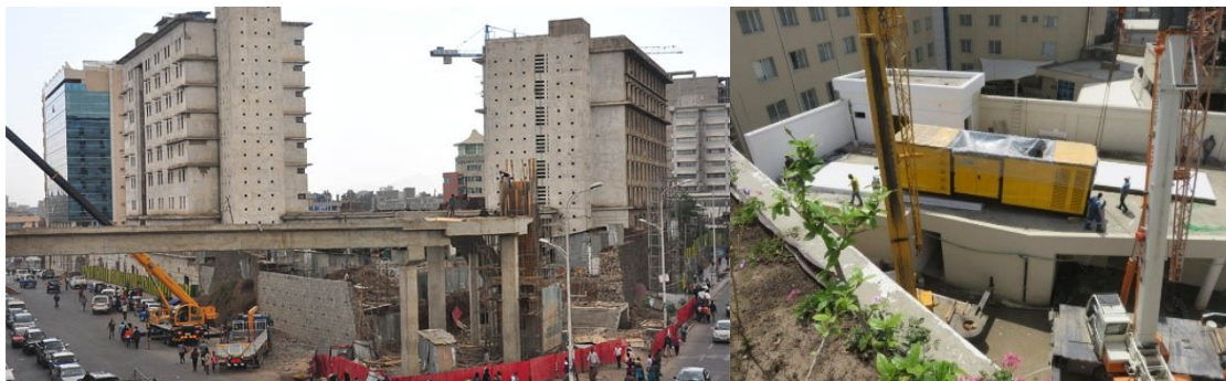
Figure 49 Top view of Hyatt Regency Hotel Project, ASB Hotel Properties PLC, green roof and balcony gardens (under construction).
