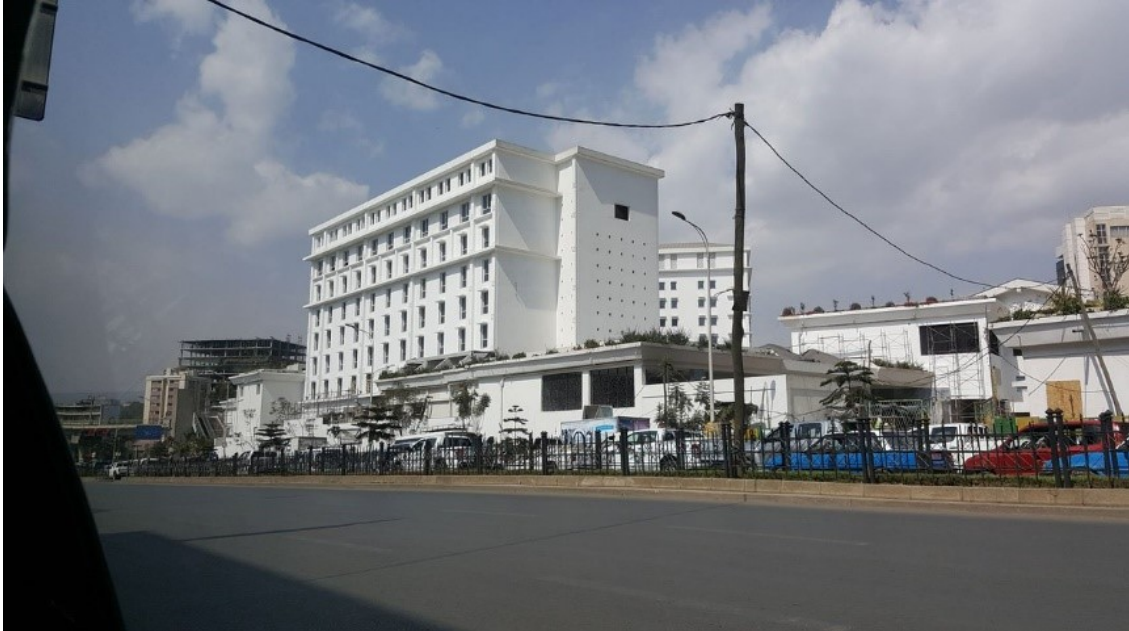
Figure 48 View from street Hyatt Regency Hotel Project, ASB Hotel Properties PLC, green roof and balcony gardens (under construction)
