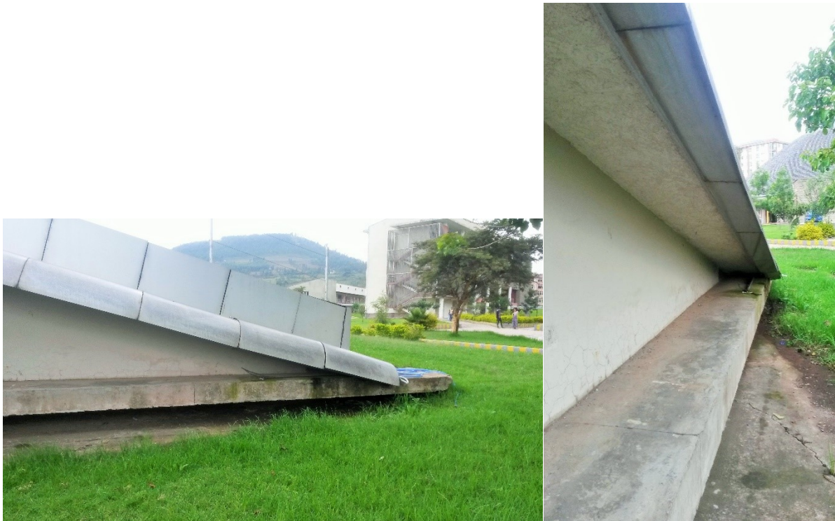
Figure 27 the Library seen from side walls, connections, and joints that need a specific design detail. Image source: site visit.
