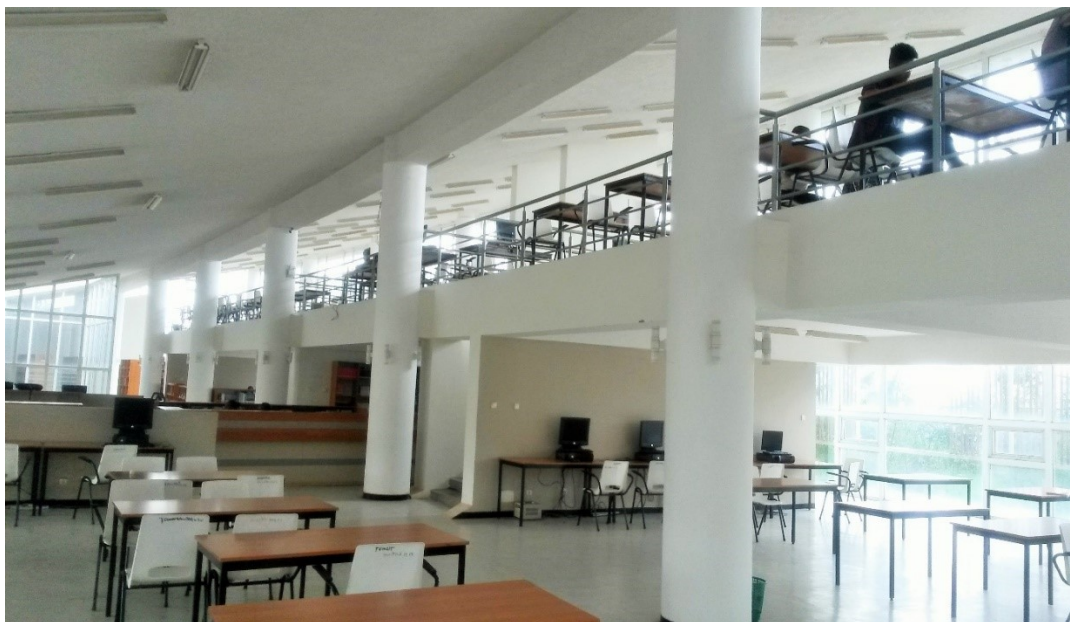
Figure 34 again reading area and Hallway: Roof slabs similarly being in clear condition same as conventional roofs .image source: site visit.
