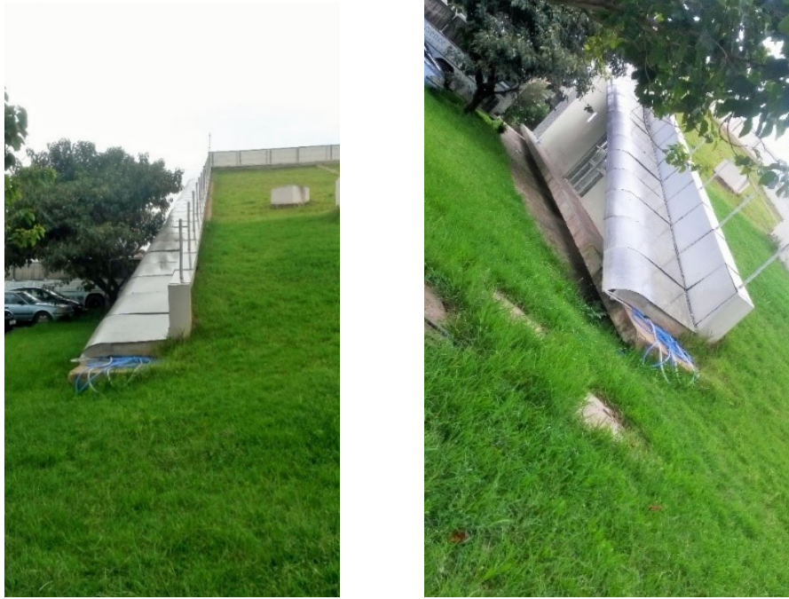
Figure 25 Special connections and joints on the green roof that needed specific green roof details to avoid problems such as leakage and related issues. Image: site visit.
