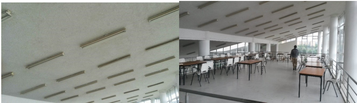
Figure 31 Roof slabs being in clear and clean manner (same as conventional roofs without green roof). Image source: site visit
