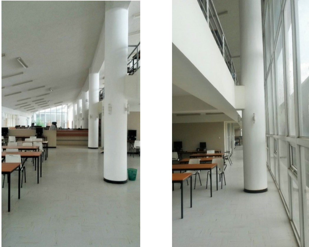
Figure 33 Hall way Roof slabs: similarly being in clear and clean manner same as conventional roofs without green roofs. Image source: site visit
