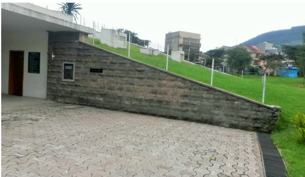
Figure 28 the Library seen from side walls, connections, and joints that need a specific design detail. Image source: site visit
