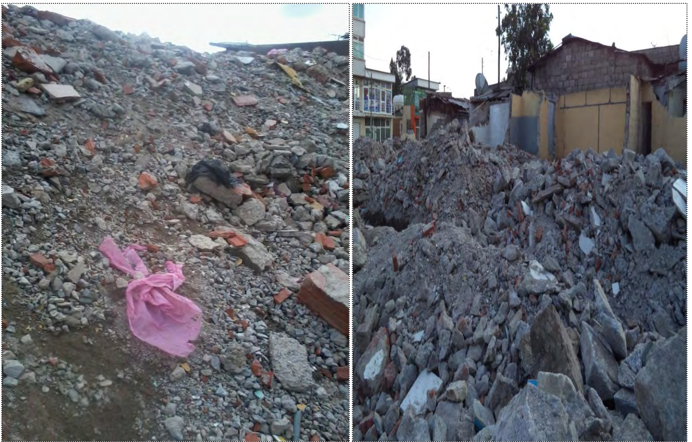
Figure 5.14: Improper handling of debris on site without disposal in front of AU
