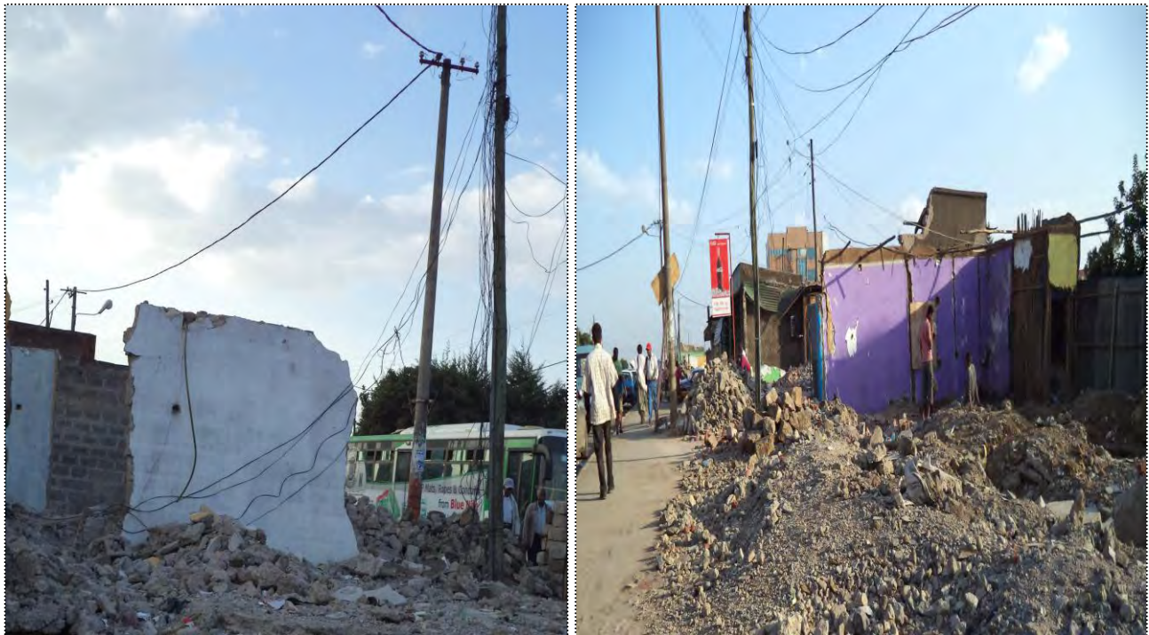
Figure 5.11: Demolition without electric cable disconnections around Bulgaria embassy
