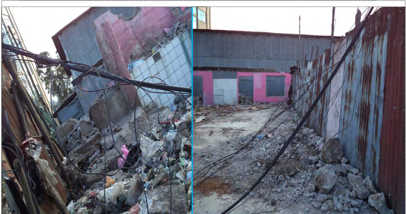
Figure 5.12: Improper disconnections of water, telecommunication and electric cables
