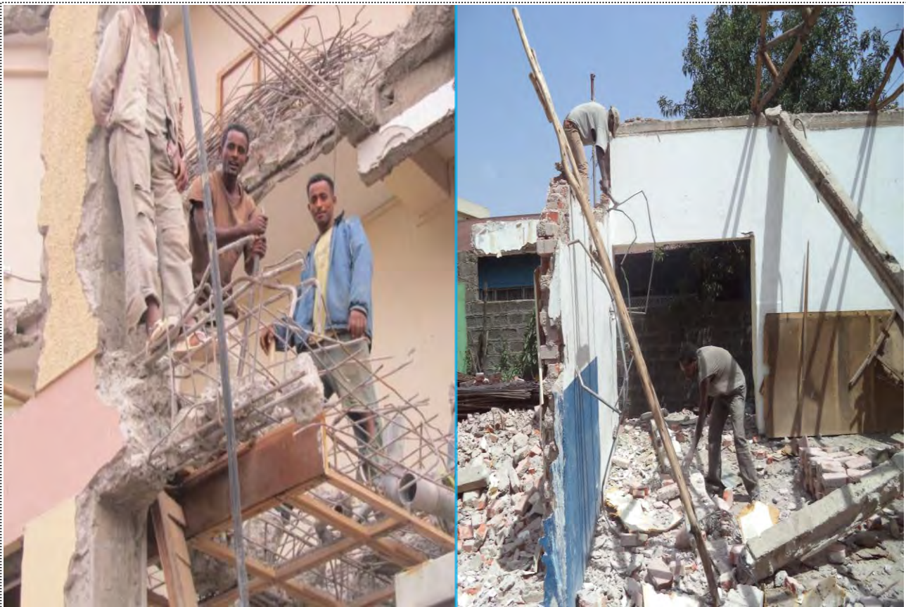
Figure 5.17: Demolition workers without wearing personal safety equipment in Axum Hotel and around Mexico square
