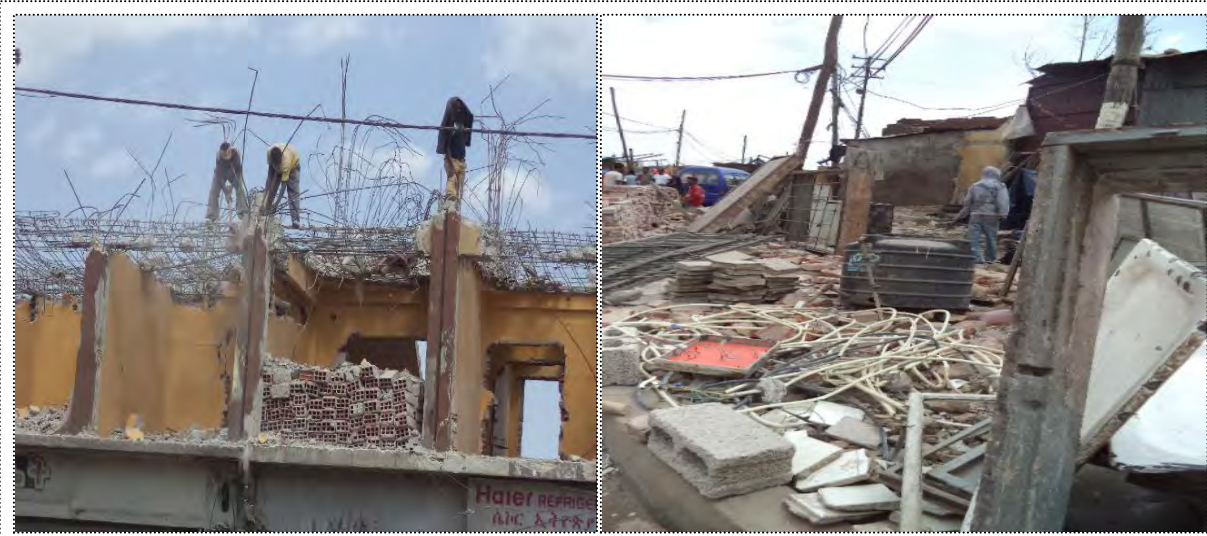
Figure 5.3: Demolition workers without personal protective equipment ( American Gibi )
