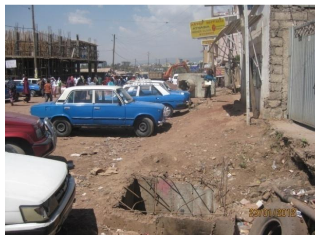
Photo 12: Manhole left open with exposed rebar (Bole Rwanda- Bole Michael Road)
