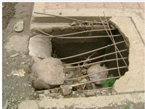
Photo 8: Damaged manhole cover on the walkway poor workmanship (Mekanisa-Jemo road)
