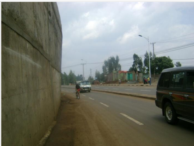
Photo 7: Retaining wall tilting, error likely in erecting formwork during construction (Wingate - Asko Bridge Road Project)
