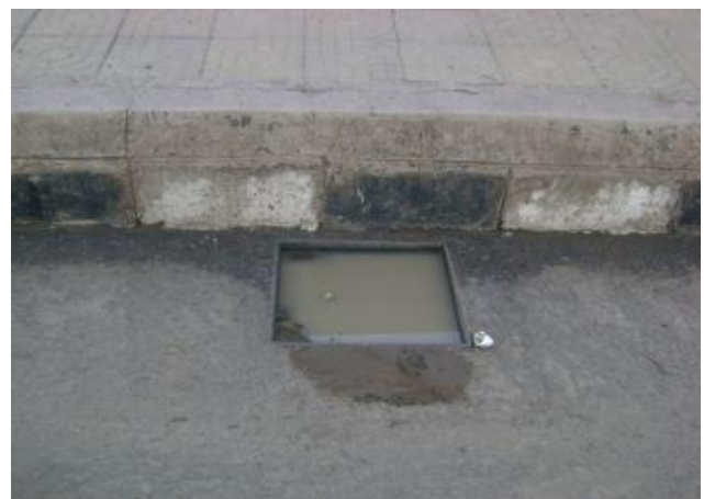
Photo 10: Clogged gully manholes resulting in pond water (Wolo sefer-Gotera Road).
