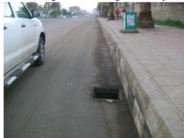
Photo 9: Storm water entry gutters gully manhole cover stolen (Wolo sefer-Gotera Road)
