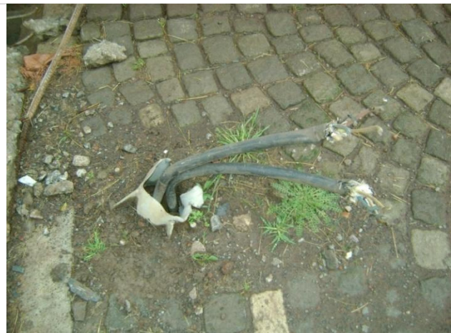
Photo 6: Damage to street light pole leaving possibility for electric hazard (Mekanisa-Jemo road).
