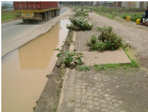
Photo 5: Man Hole being clogged & not functional (Mekanisa-Jemo road)
