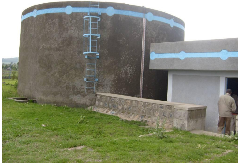
Figure 5: 300m 3 Service Reservoirs in Fitcha at Torban Ashe
