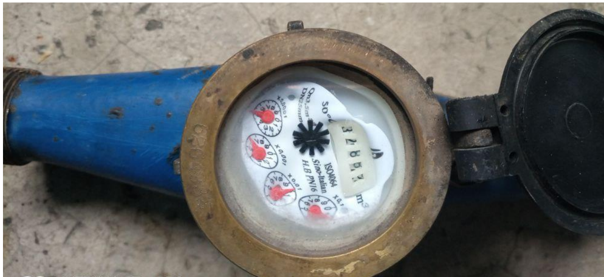
Figure 15 Shrinkage inside a water meter
