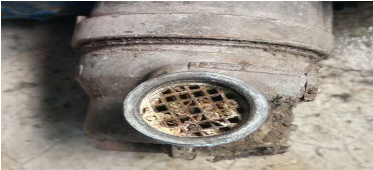
Figure 24 Partial blockage of inlet strainer
