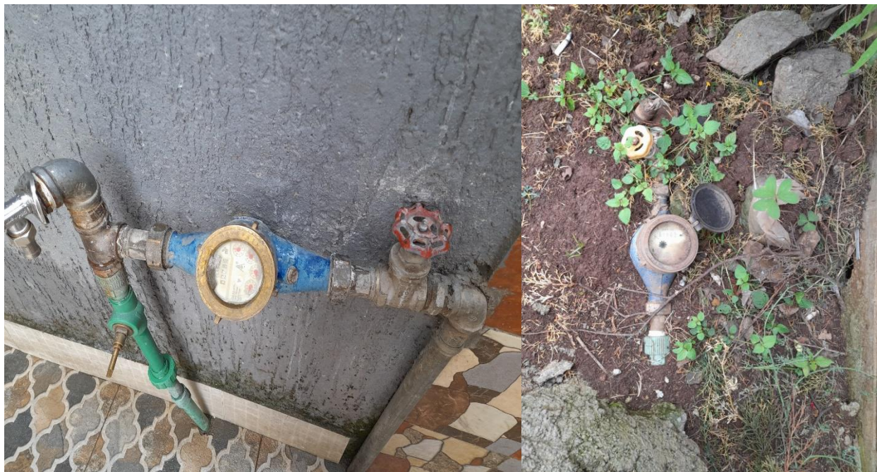
Figure 23 Incorrect Meter Installation
