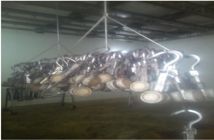
Figure 2: Nonfunctional cooling room in Adama municipal abattoir
