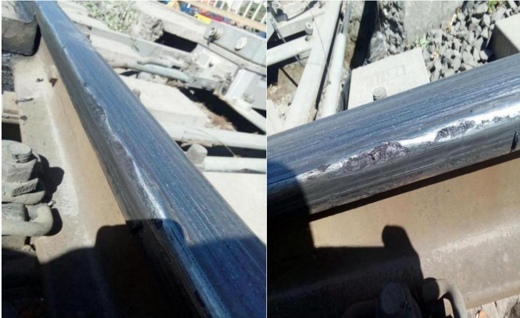
Fig 1- 2 Wear on main line truck gauge corner of AALRT
