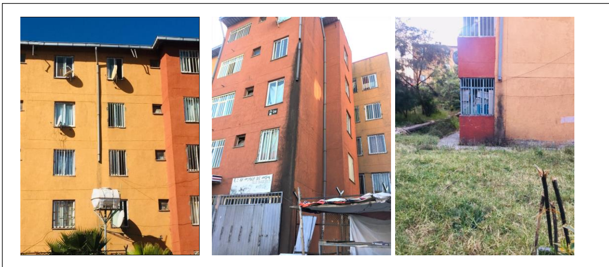
Figure 39: Drainage line needing maintenance
