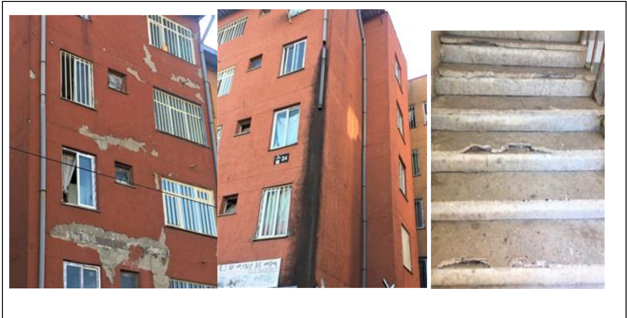
Figure 34: Physical deterioration of the building parts
