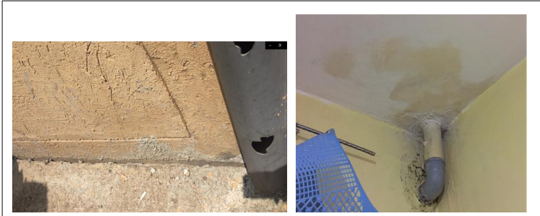
Figure 30: Dampness cause in the building
