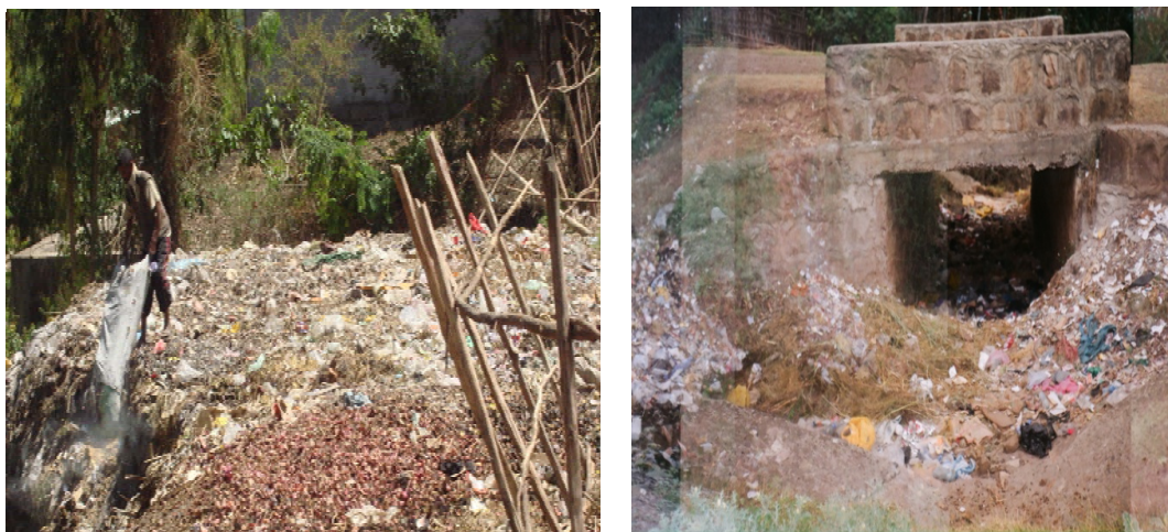
Picture 4.9: Partial view of informal sectors illegal solid waste disposal. Source: field survey, 2011
