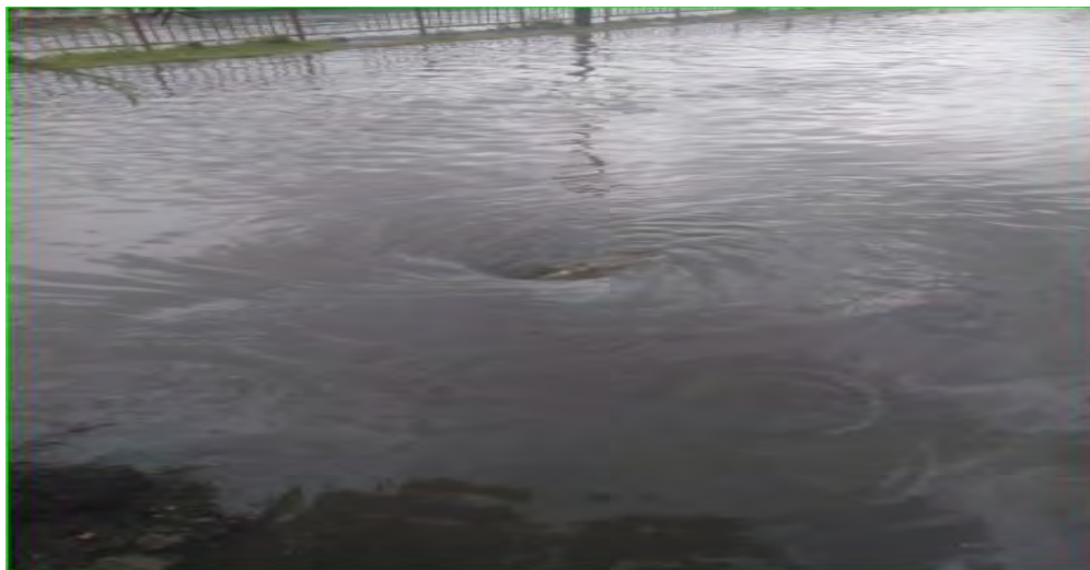
Figure 7: Photo showing under sized inlet in front of Bole International Airport
