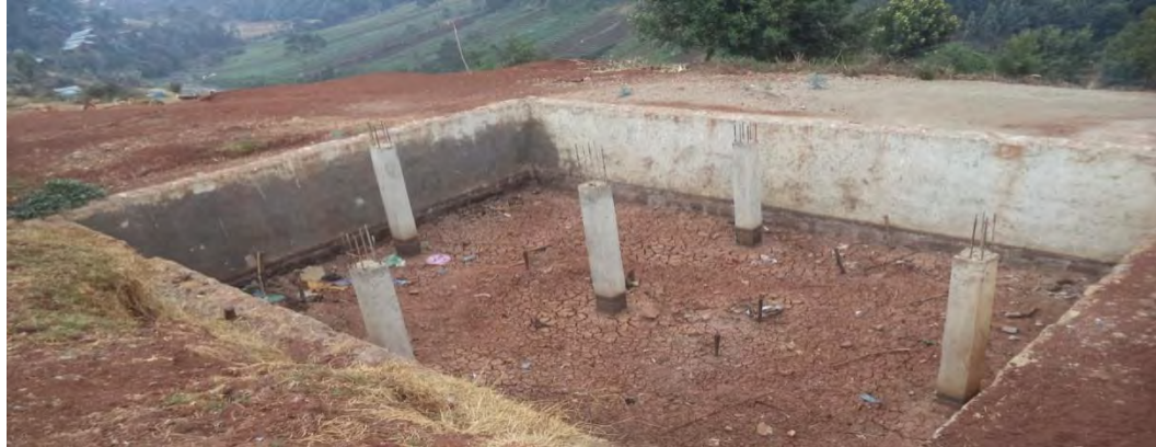
Figure 4.3: Municipality's abattoir treatment plant
