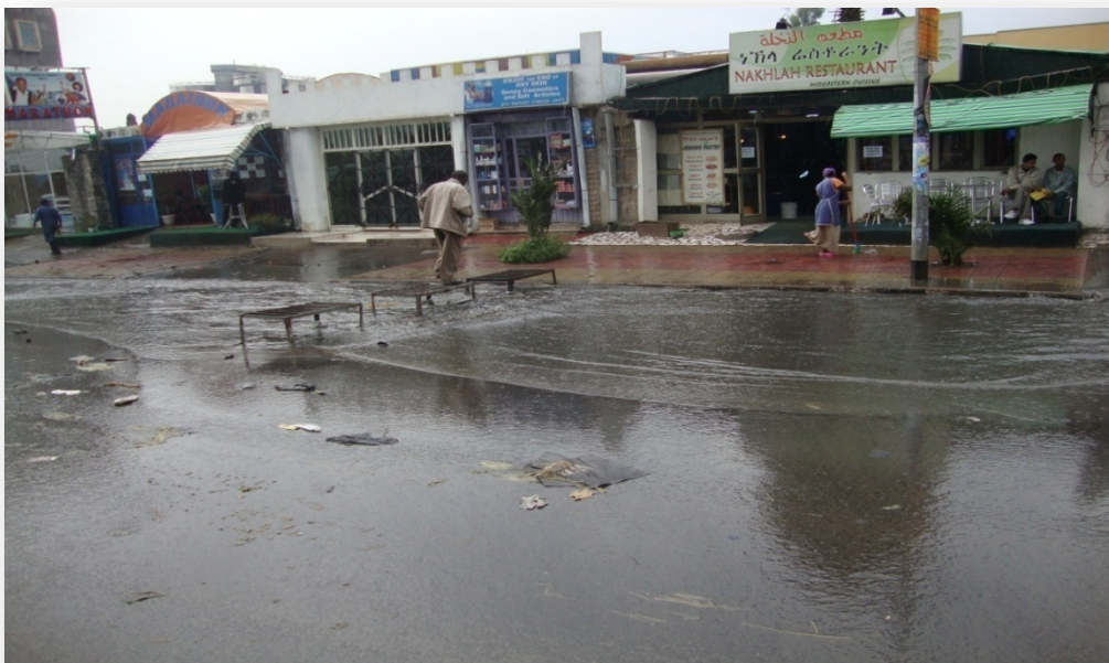
Fig 1.4) Drainage problem at Ring road
