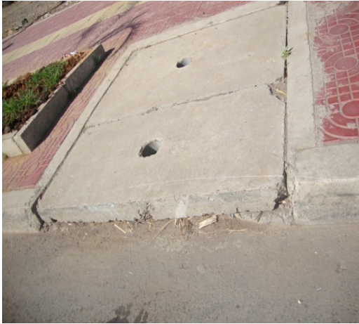
Fig 3.5 a) Inlet blocked by silt and garbage
