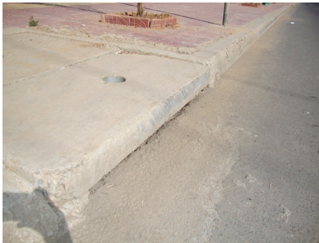
Fig 3.5 c) under designed curb height (12 cm) and small inlet opening
