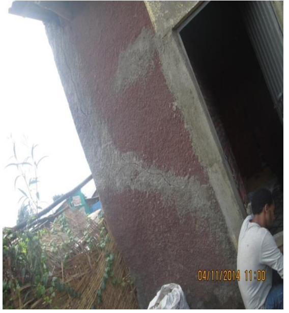
c. Wall cracks due to edge lift.
