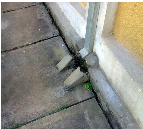
c. Displaced walkway
