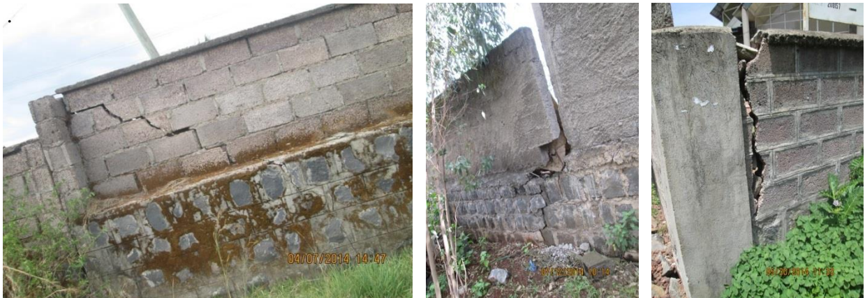
Figure 4.9 Sample pictures of damaged fences
