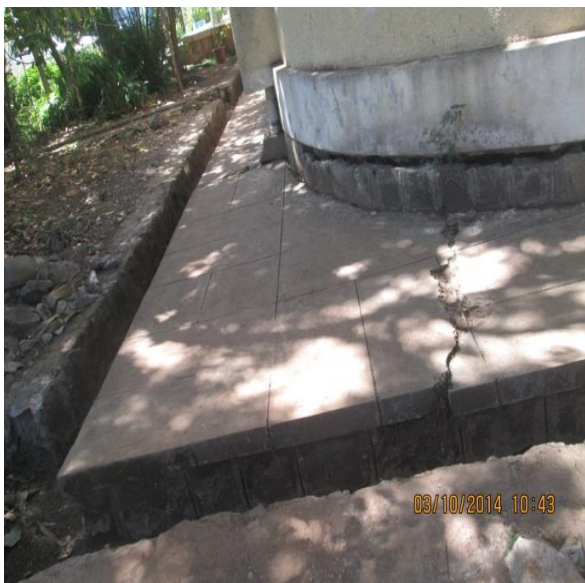
a. Cracks, vertical and horizontal movement
