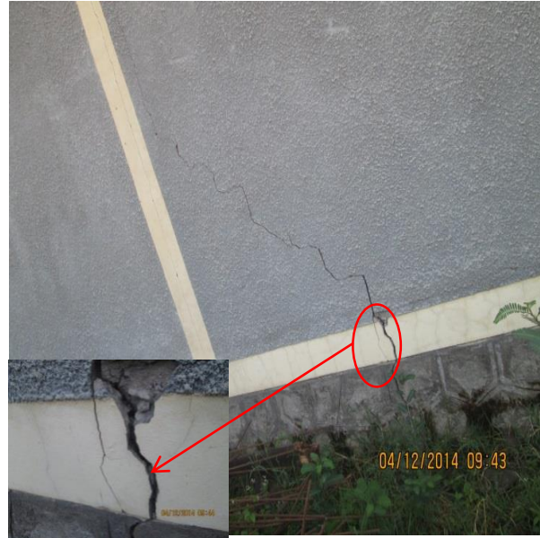
c. Masonry crack extended to grade beam and HCB wall.
