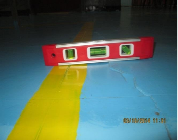
a. Bulged floor
