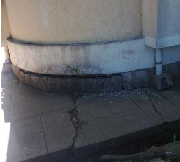
a. Cracked pavement and separation of masonry foundation from grade beam
