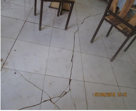
b. Cracks in different direction
