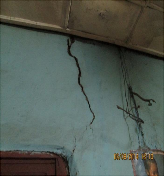
b. Cracks starting from door corner.
