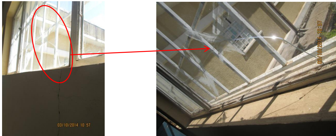
f. Diagonal cracks extended to glass from HCB wall
