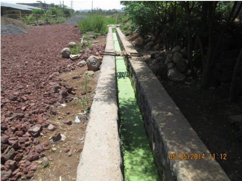
Figure 5.2 Gray water accumulated in road side ditch
