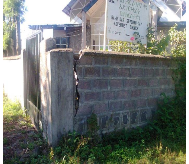
b. HCB fence wall separated from corner column
