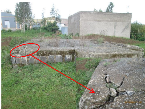
d. Seriously damaged masonry foundation, grade beam and floor slab.
