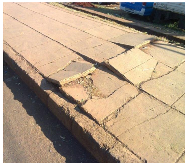
d. Bulged and disintegrated road side walk way
