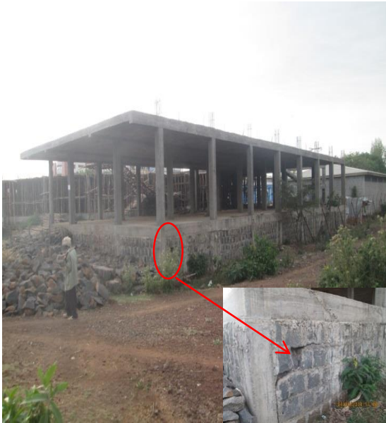
b. Building under construction and masonry started cracking.
