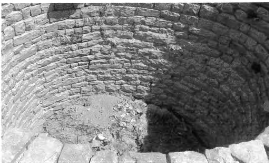
Plate 4.3: Unfinished pond due to lack of cement (Mai-Quiha)
