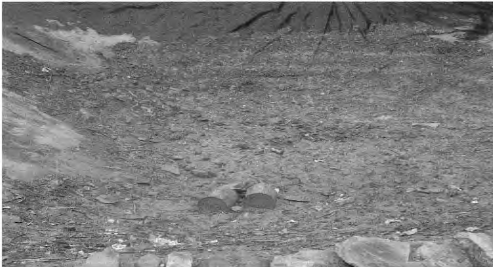
Plate 4.1: Plastic lined pond constructed without a silt trap (Negash)
