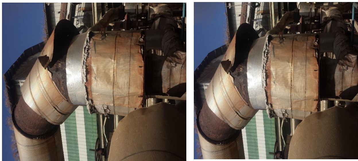
Figure 4. 5: Some of main steam lines with deteriorated insulation
