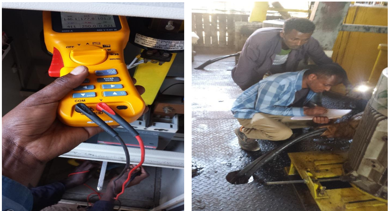
Figure 3. 20: During measurement of motor input power and nameplate data collection
