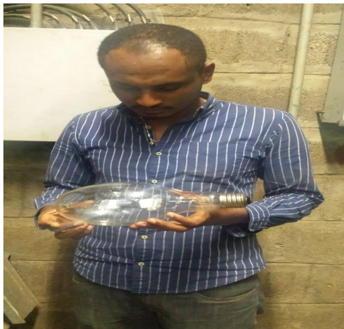
Figure 3. 27: 400w mercury vapor lamp in boiler house
