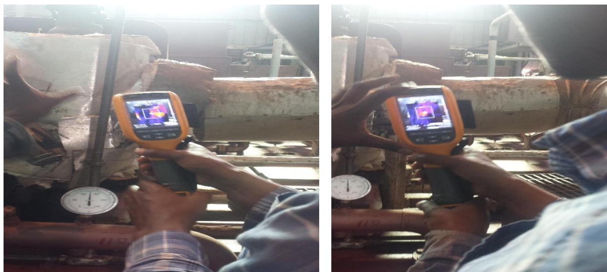
Figure 4. 6: Photos during measurement of steam lines surface temperature
