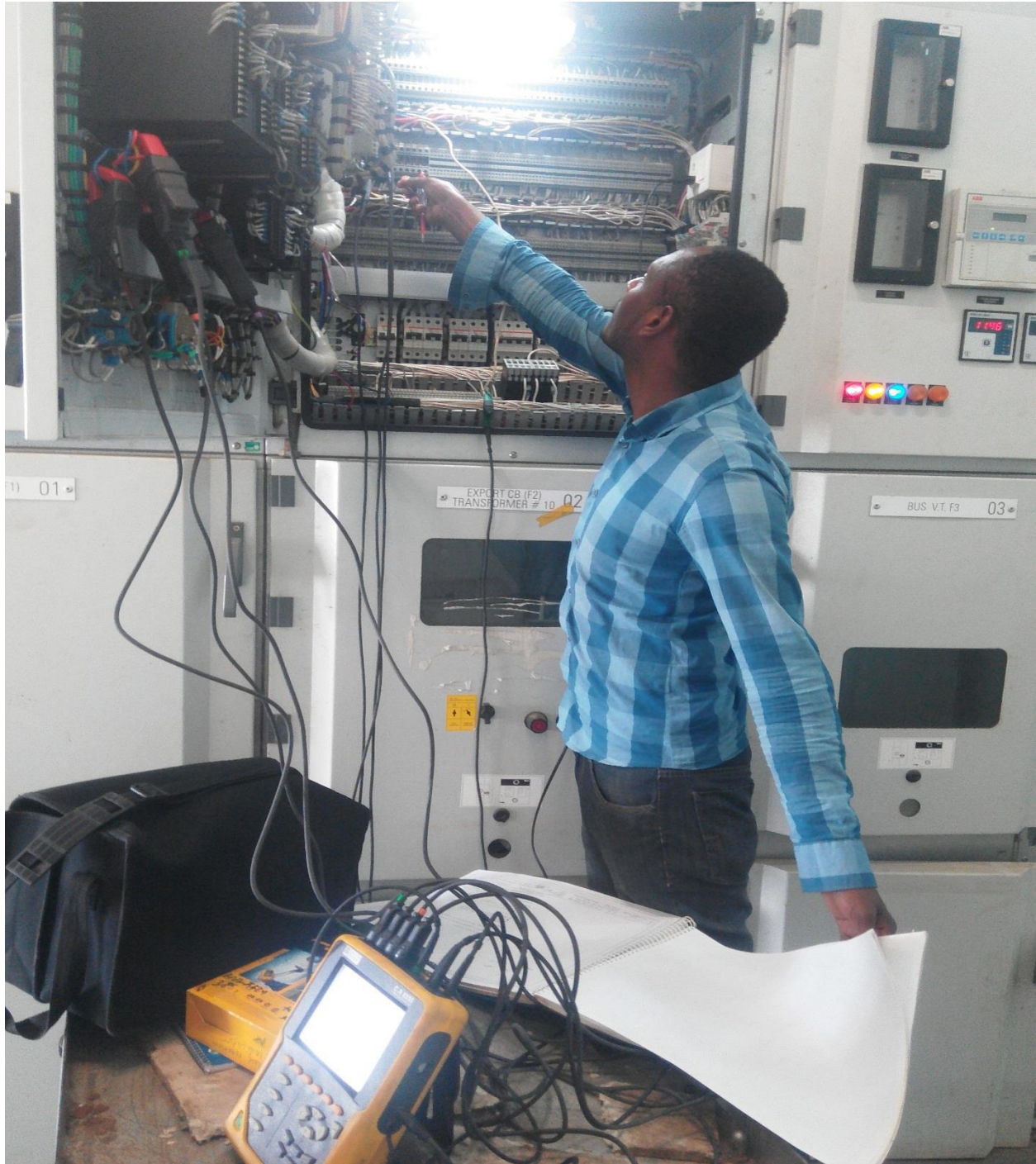
Figure 3. 4: During Measurement of power and power quality on 11kV at HT side.
