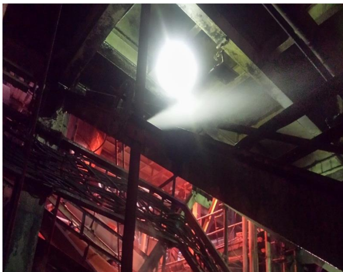
Figure 4. 11: Observed steam leakage in process plant
