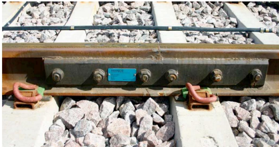
Figure 1.1 A newly installed insulated joint on The West Coast Line in Sweden [23]
