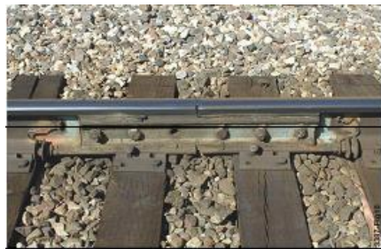
(i) Typical pull-apart of IRJ in track
