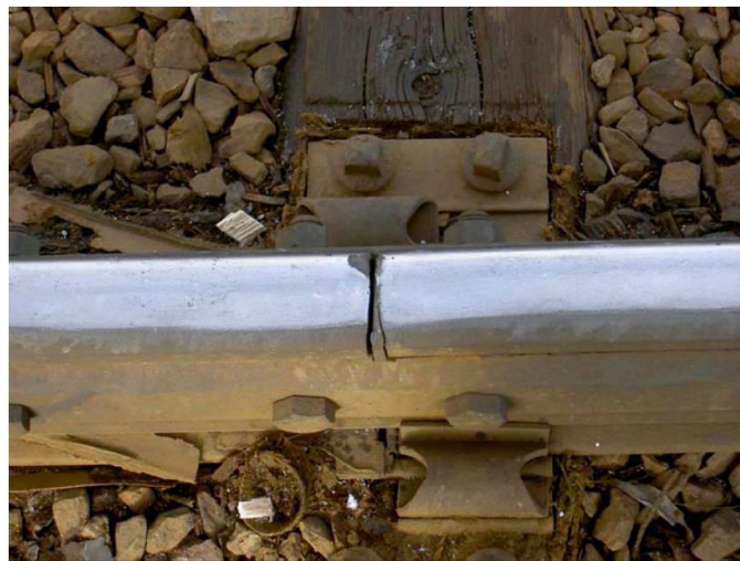
Figure 1.2: deteriorated insulated joint [24] and [25]
