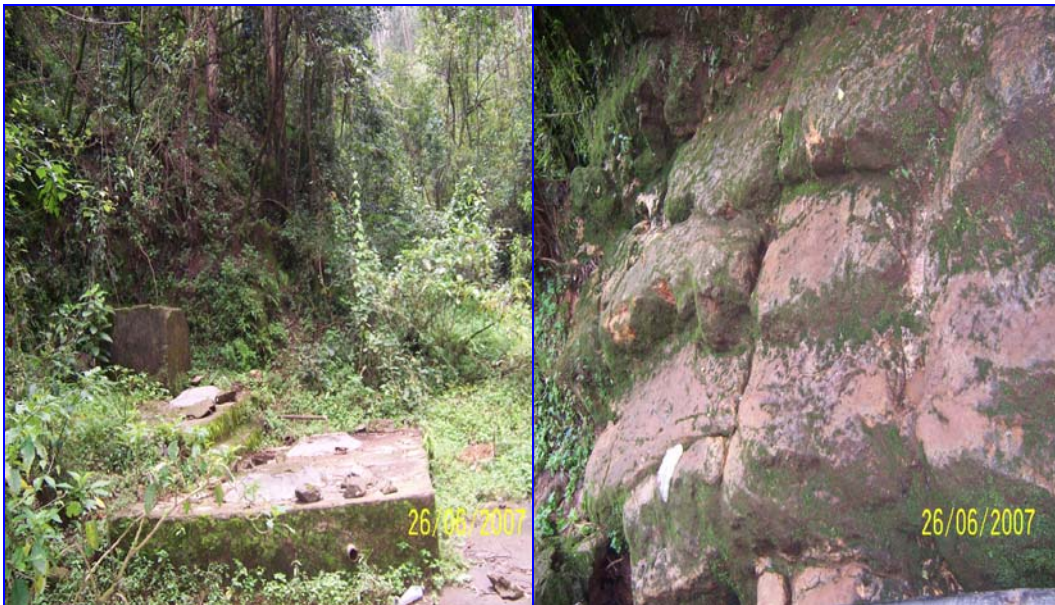
Figure 7-3: Spring capping structure (left), Weathered and fractured rhyolite (right)
