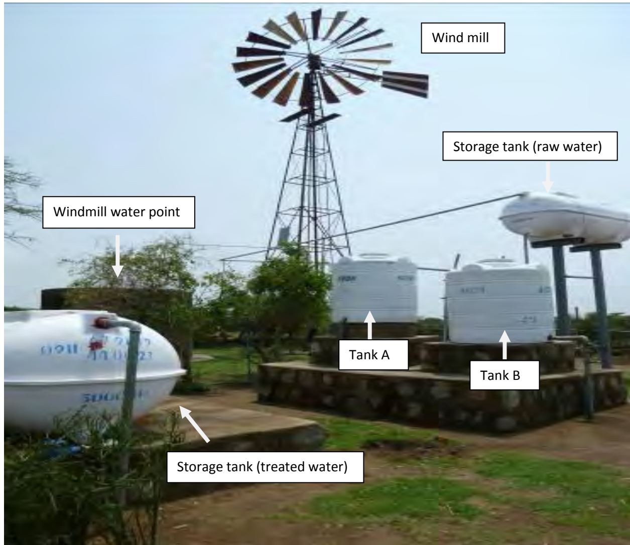
Figure 10. AO community defluoridation pilot plant implemented in Tuchigragona.
