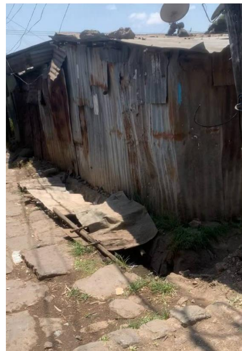
Figure 4.32. Open sewer line for rain water and sewage waste is located adjacent to or near every housing edge with heightened bad smell
