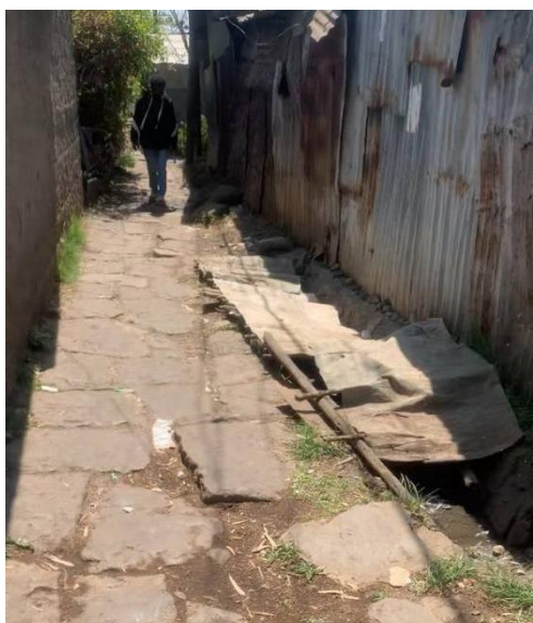
Figure 4.20. Drainage line covered by dwellers to avoid smell
