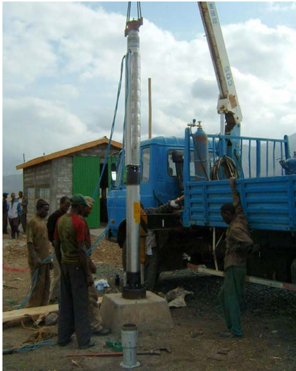
Figure 25 Pump installation for irrigation
