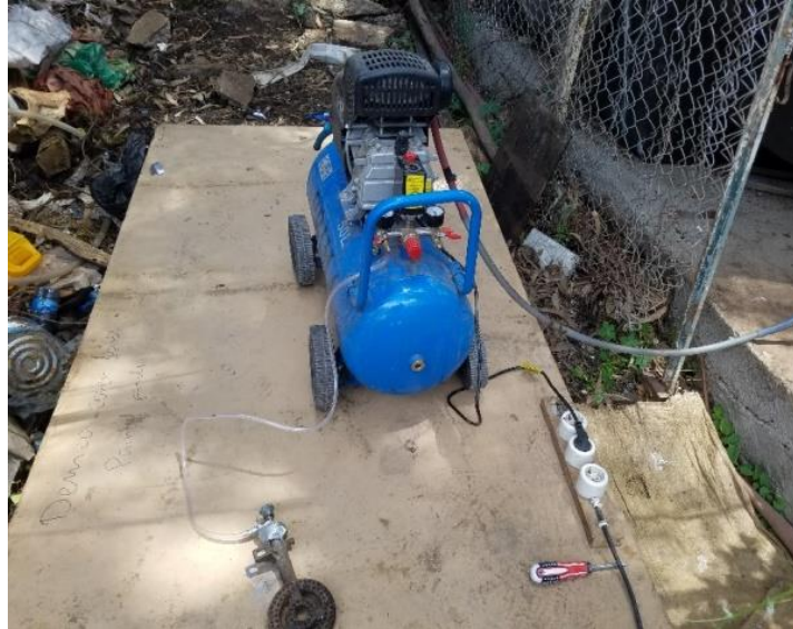
Figure 53 Biogas compressor connected to line on a gas stove
