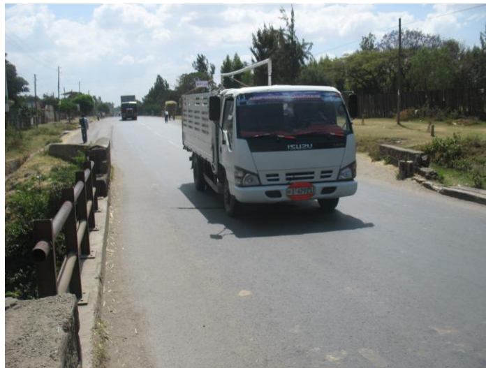
Figure 14. Awade Godu bridge damaged post and rail system
