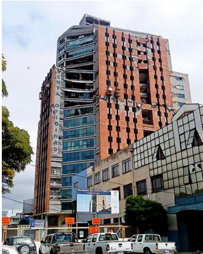
Figure 2.2 Partial collapse of o'Higgins office tower in Chile [2]
