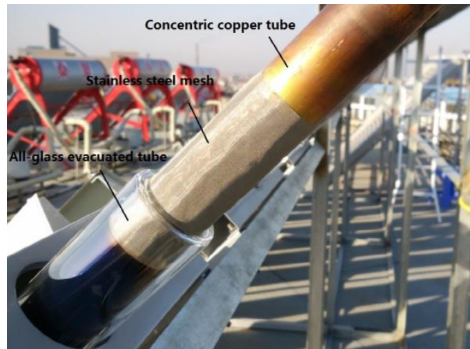
Figure 2-19: Photograph of CPC collector with coaxial pipe (Wang, Li and Liu, 2015)
