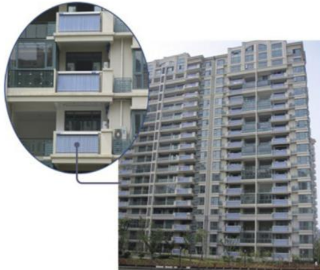
Figure 2-4: Appearance of the evacuated tube solar water heater integrated in the building (Li, Dai and Wang, 2015)
