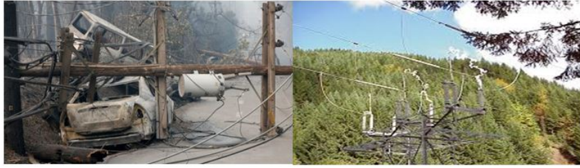
Figure 1.2: Distribution system failure due to different causes (Source: google images)
