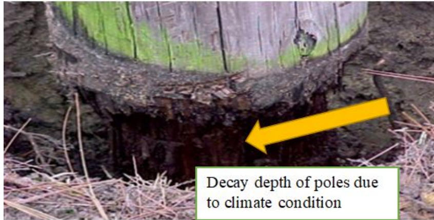
Figure 2.3: Decay of distribution pole due to climate influence [17]
