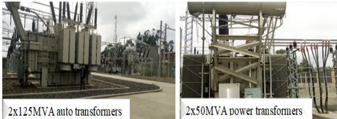
Figure 3.2: New substation transformers
