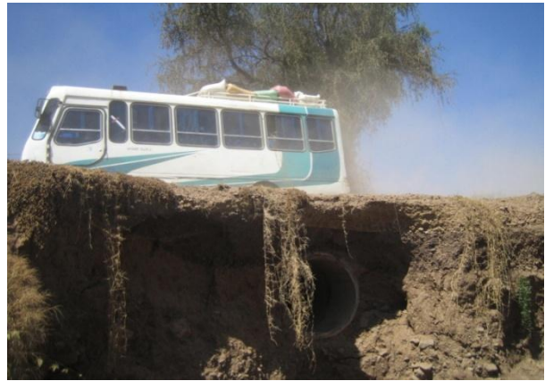
Figure 5-2: Poorly provided diversion road around structure construction area
