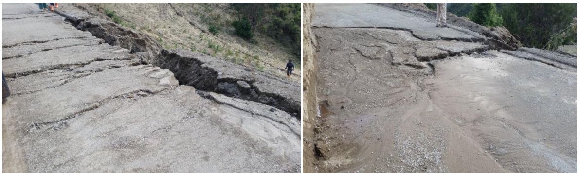
Plate:5.2 Damage on subgrade soil caused by rainfall which indicate importance of
