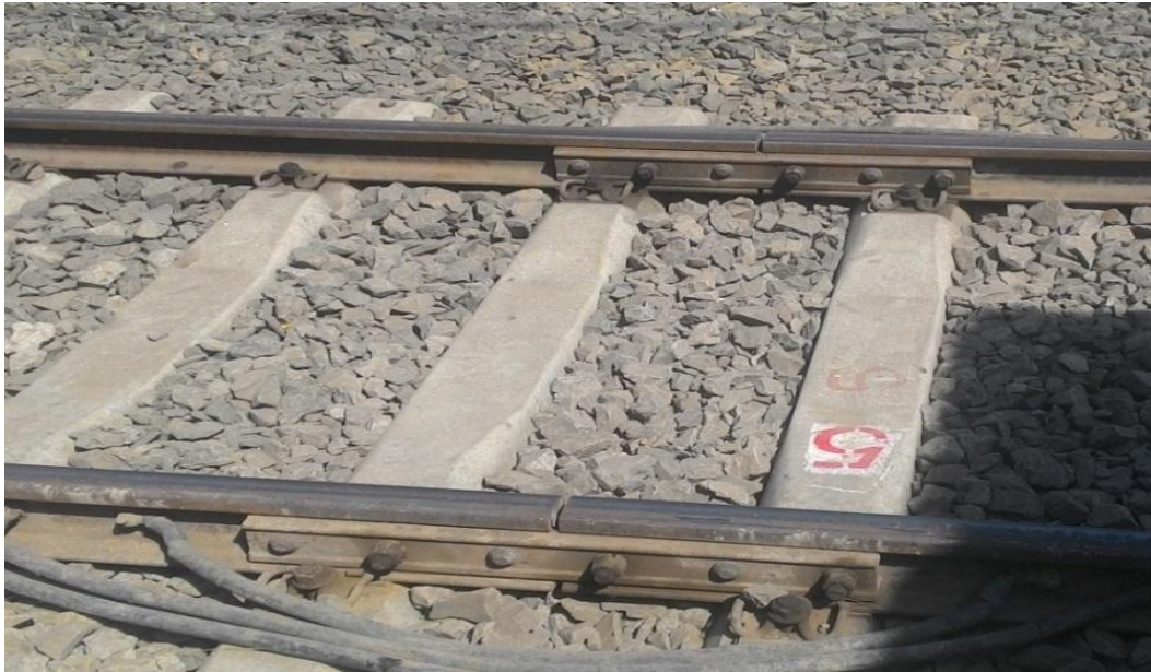
Figure 5-1 Bolted rail joint, Addis Ababa LRT
