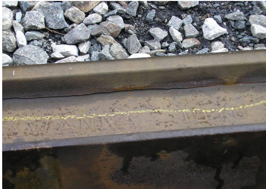
Vertical Split Head Crack Out in Head/Web Fillet Area
