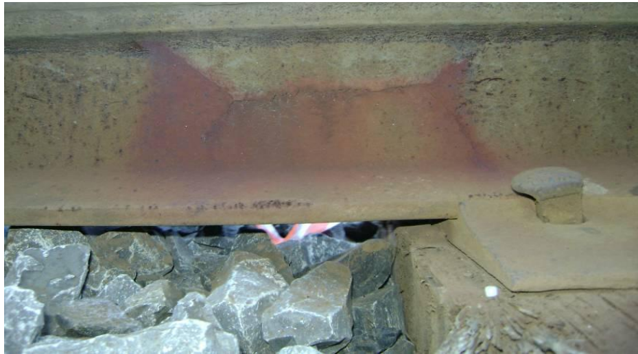
Split Web Defect Showing Bleeding Condition along Crack Development
