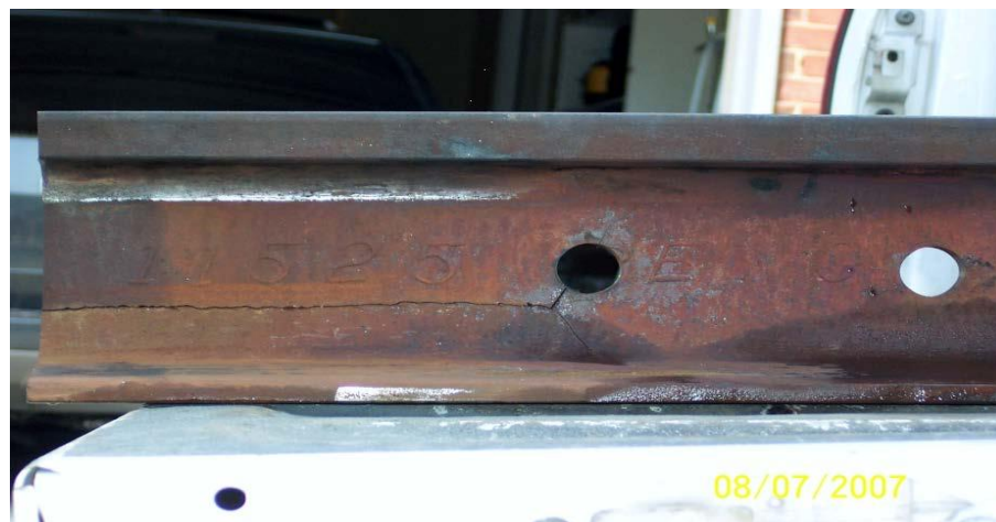
Bolt Hole Crack Originating in Lower Quadrant with Significant Progression
