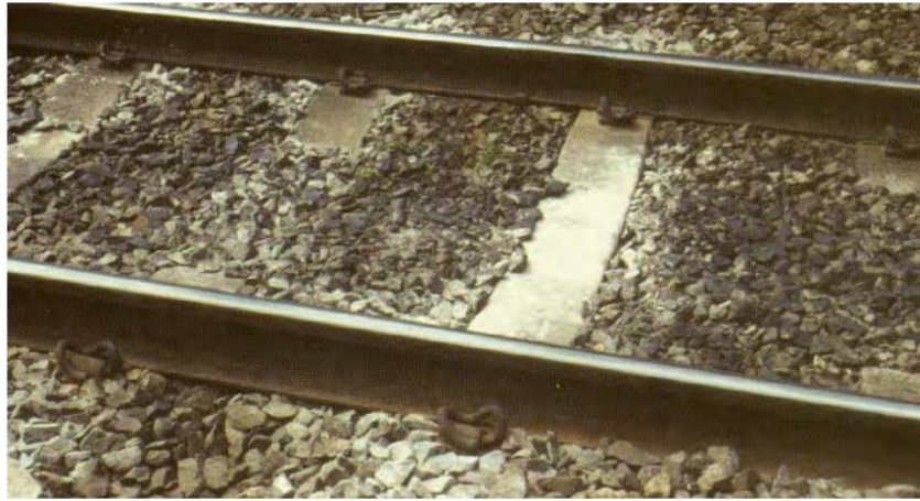
Figure 2.3.2 Voids below concrete sleeper identified by white powder around the sleeper (Cope and Ellis, Calla C., 2003)
