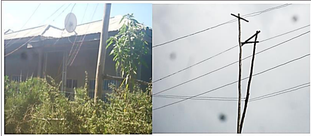
Figure 4.18 Informal connections of electric wire from a single electric meter to neighborhoods
