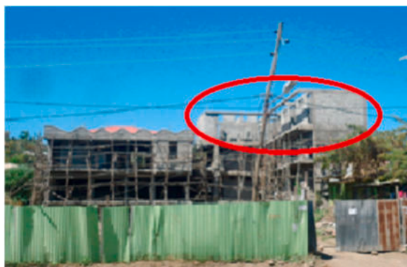
Fig. 8. Unauthorized rooms under construction on the roof of the building in the town at Gonder Ber . Photo by Author (2019).
