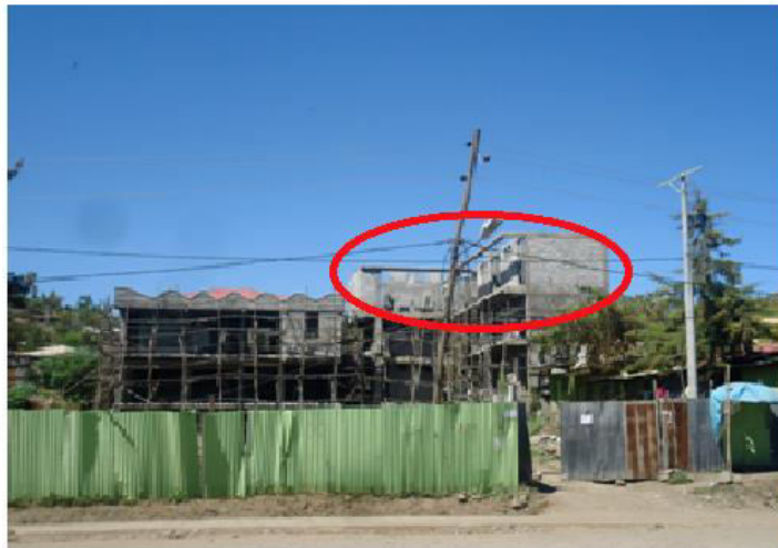
Figure 4.6 Unauthorized floor and rooms extension in the town at Gonder Ber
