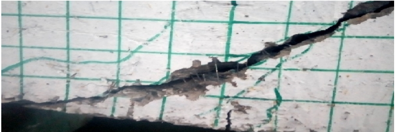
Fig 5-11 S50VF1%C after failure (close up view)
