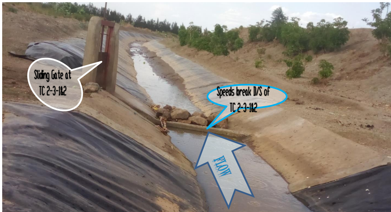
Figure 4-3: Existing Speeds Break at Offtake TC 2-3-1&2 used as cross regulator
