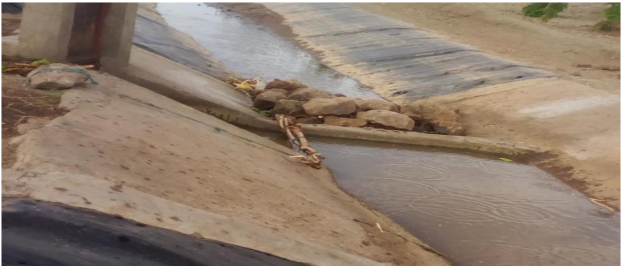
Figure 7-2: Waterlogged boots as a cross regulator constructed by irrigators/farmers
