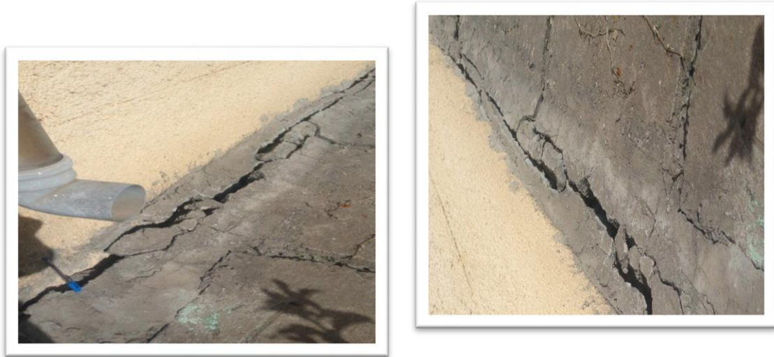
Figure 2. 7 pictures of building affected by expansive soil
