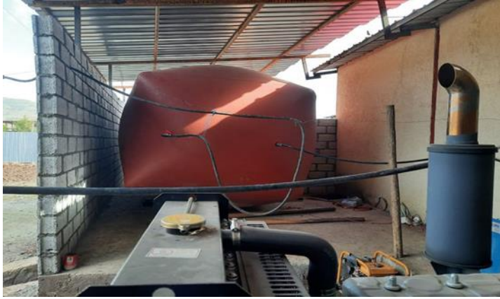
Figure 7 Abio-digester plant in Zagol Milk and Dairy farm.
