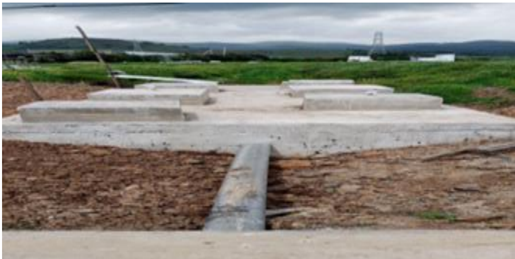
Figure 8 Waste treatment plant in Zagol Milk and Dairy farm
